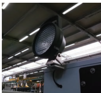
Light on pump side
